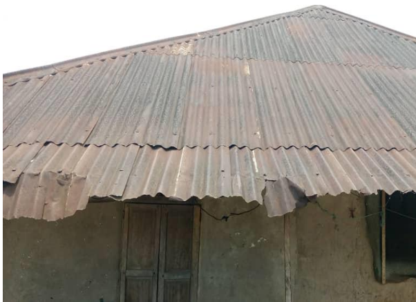
Figure 4: Roofing condition at Bodo
